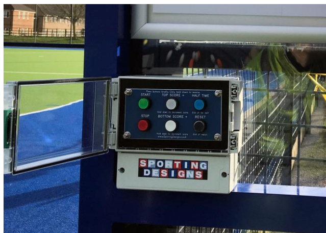
The fixed control unit
